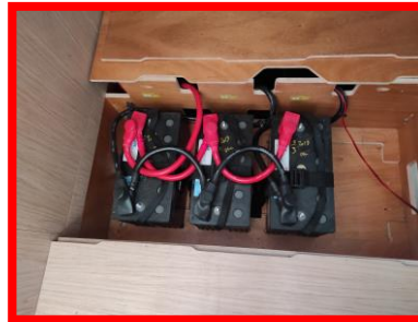
Both Sets of Batteries are located under the beds.
