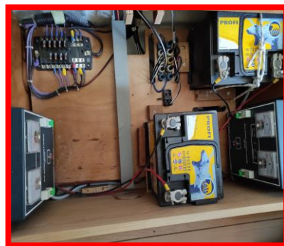
GMDSS battery and charger, located under the main bench.
